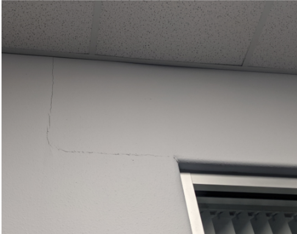
Figure 5 – Gypsum Wall Crack at Interior Wall
